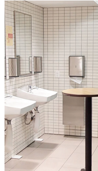
Stacked bond wall tile in the existing restrooms Photo from the Matterport virtual tour
